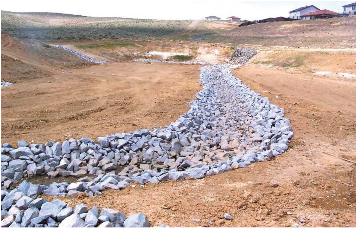
Figure 3: Our design standard of a cobble line low flow channel for detention/retention basins.
